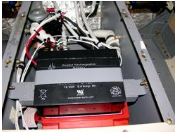
Auxiliary battery installation
