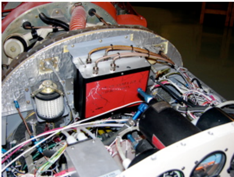
The Plasma III controllers were mounted on the firewall. Spaciousness is not a virtual of the RV-4. Every square inch is precious.
